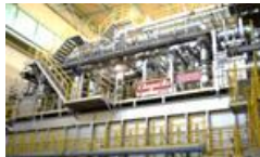
Energy-saving heating furnace that uses regenerative burners
