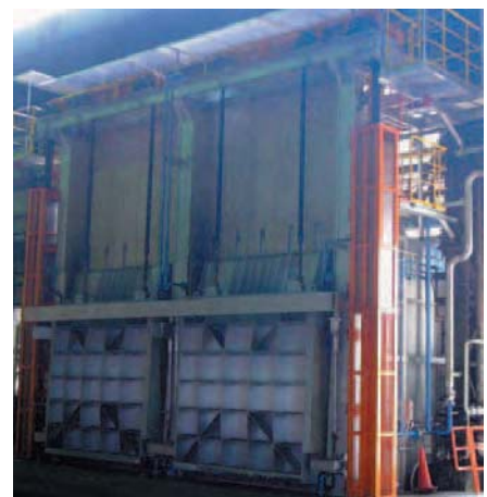
A newly installed reheating furnace also runs on LNG.
